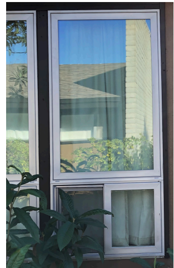
NON-Compliant Replacement Window - mullions too thick
